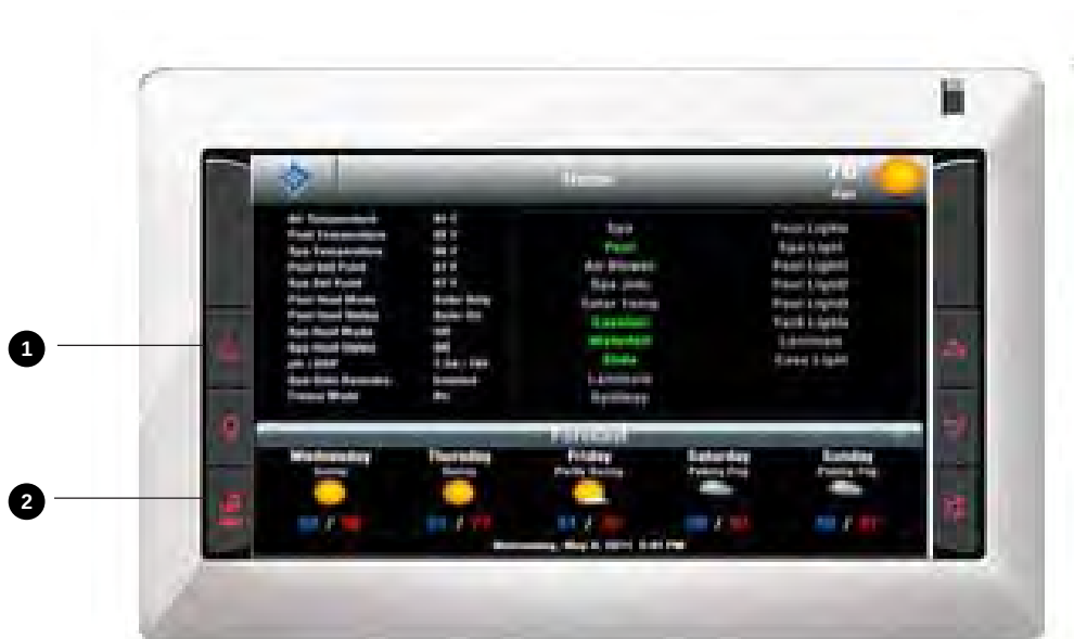
In-Wall Touch Screen (Controls)
